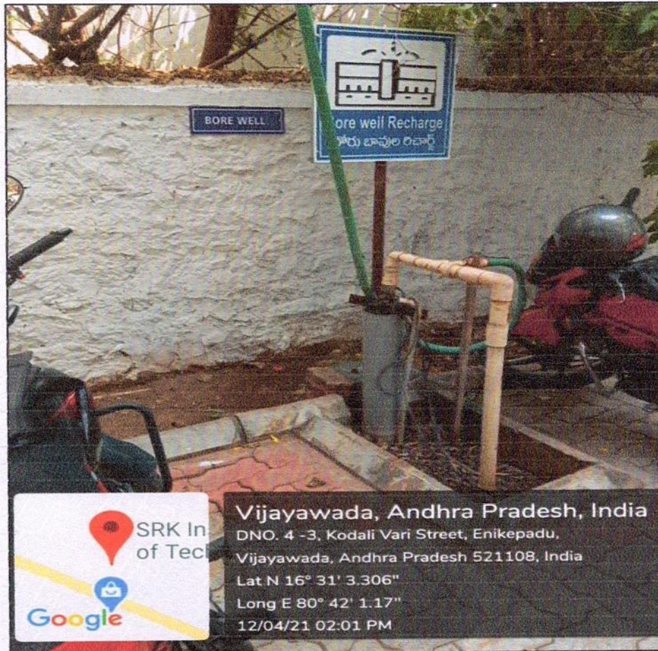
Bore well recharge using rainwater
